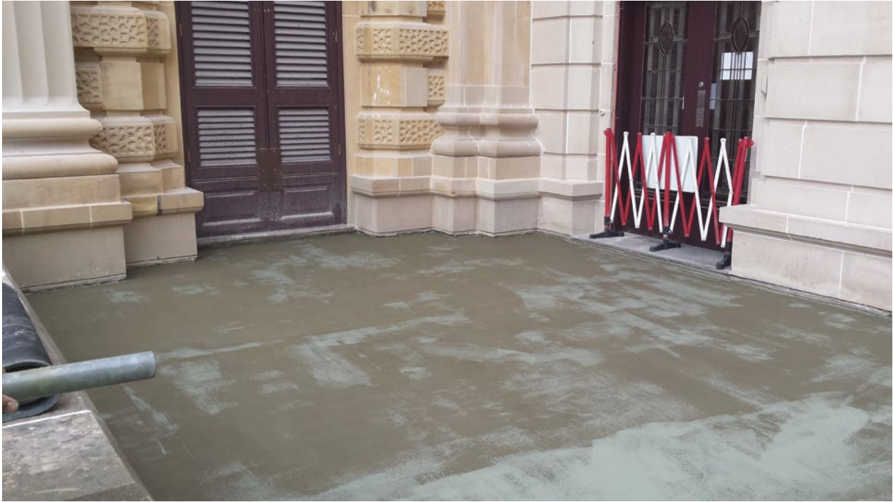
A waterproofing membrane was laid beneath the new bluestone pavers. This helps to eliminate water ingress into the kitchen beneath
