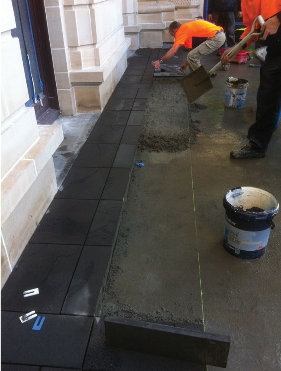
Bluestone pavers are laid in a pattern that reflects the original underneath
