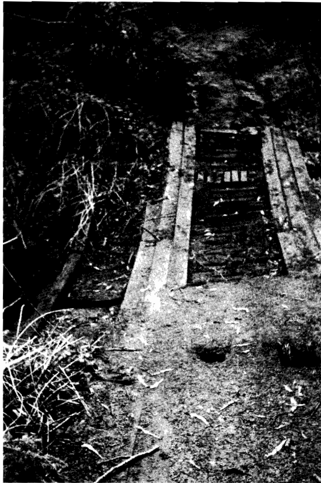
Unsafe bridge which has resulted in the closure of a major fire access track.
