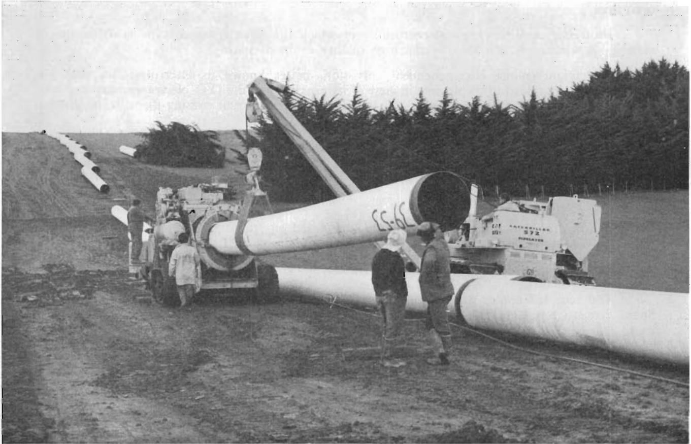
Hydraulically operated bending machine forming pipes to suit change of grade. All pipe bending was carried out in the field to the required angle at each location.
