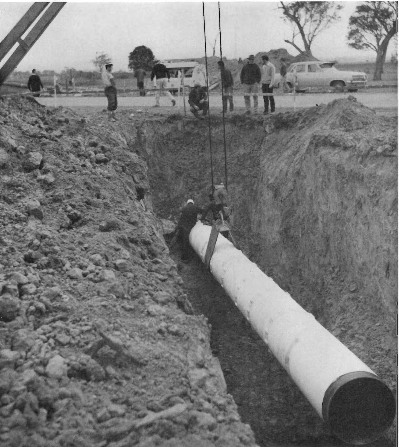
Threading a section of pipe through the steel casing bored under the Princes Highway near Flynn. The nylon casing insulators incorporate spacers to prevent the pipe coating from being damaged by the casing, and afford electrical insulation.
