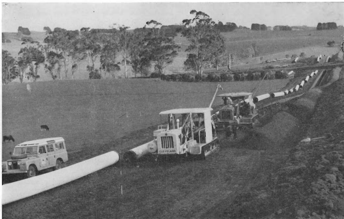
Ditching machines working in tandem near Buln Buln excavating the 7-foot deep trench after pipe stringing.
