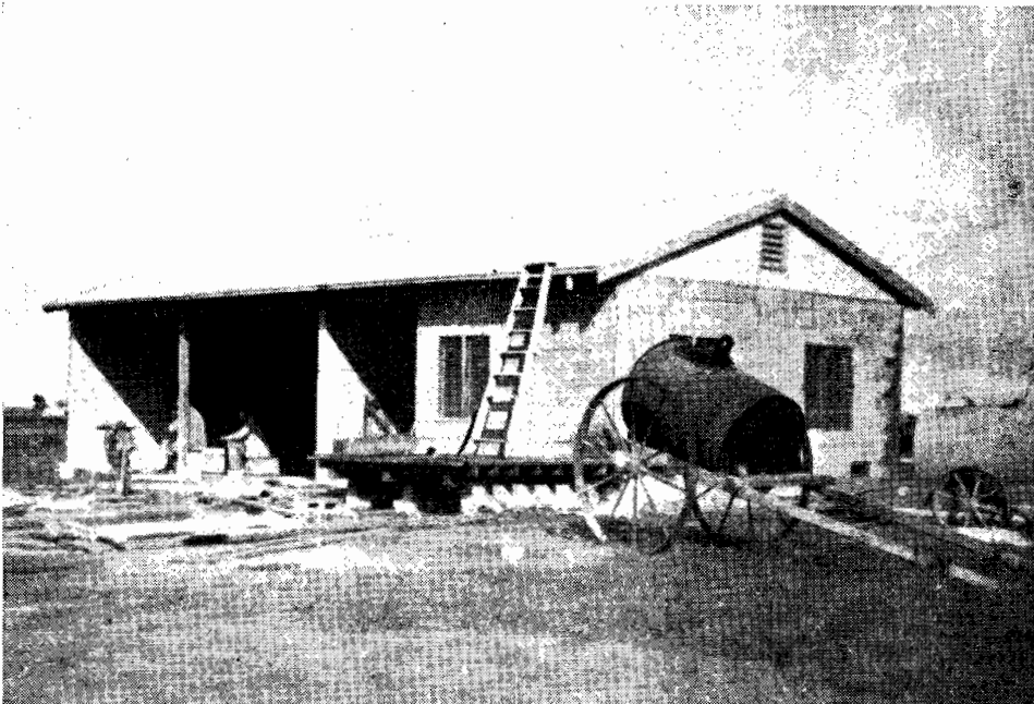
A dairy in course of construction in the Murray Valley Irrigation Settlement Area.
