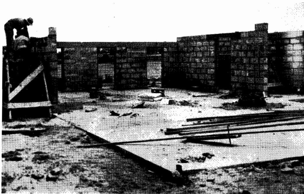
Dairy in course of erection—the concrete bricks are moulded on the site.
