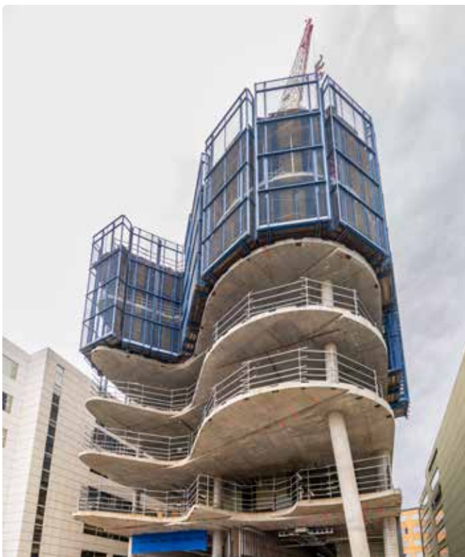
Construction on the Paula Fox Melanoma & Cancer Centre continued, with the structure reaching its highest point in June 2023.
