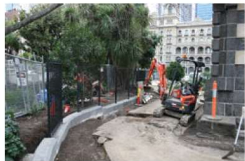
The beginning of the 2013-14 year shows promise with the south security fence works progressing quickly.
