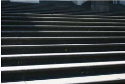
At first glance the front steps prior to the removal of the treads and waterproofing works do not noticeably show the level of damage.
