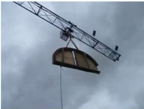
The windows were lifted out using the crane after being boarded up.
