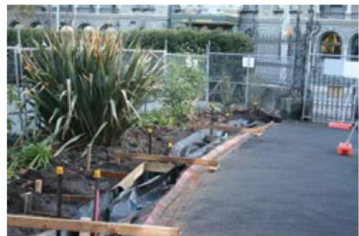
Construction works for the installation of a new fence and secure gate around the Bali Garden began on Wednesday 5 June 2013.
