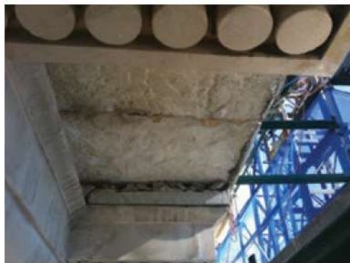
Section of the soffit where a block has been removed for repairs.
