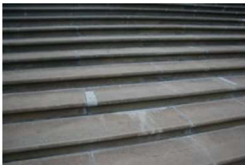
Following the replacement of the treads the areas which required repair are clearly visible and extensive, demonstrating the urgency of this project. These repaired areas will weather and colour over time to more closely match the existing stone.
