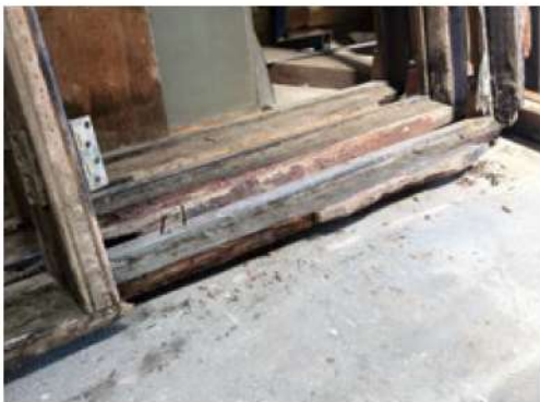
The timber on the frames was clearly worn with no sign of original paint or sealant remaining.
