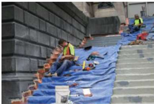
Once the treads were removed waterproofing was sprayed over the steps to seal any small cracks. Copper flashing has been installed along the length of the buttress to seal the gap.
