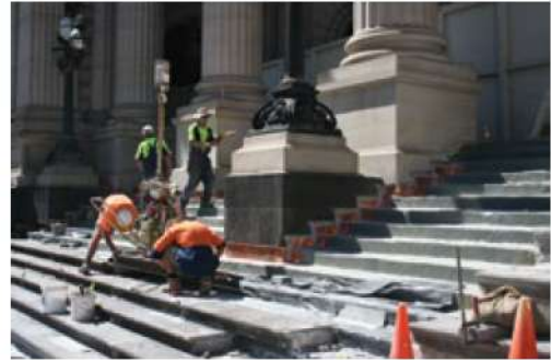
Once all the elements had been installed the treads were re-laid, having been cleaned, and in some cases, repaired.
