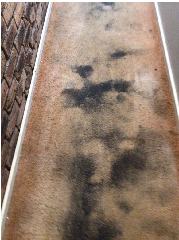
Picture of black mould on hallway carpet. More photos available.
