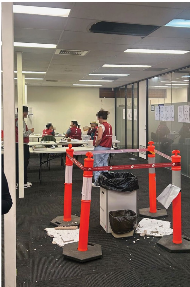
Figure 4.1 Damage to the ceiling at the Werribee District Election Office
