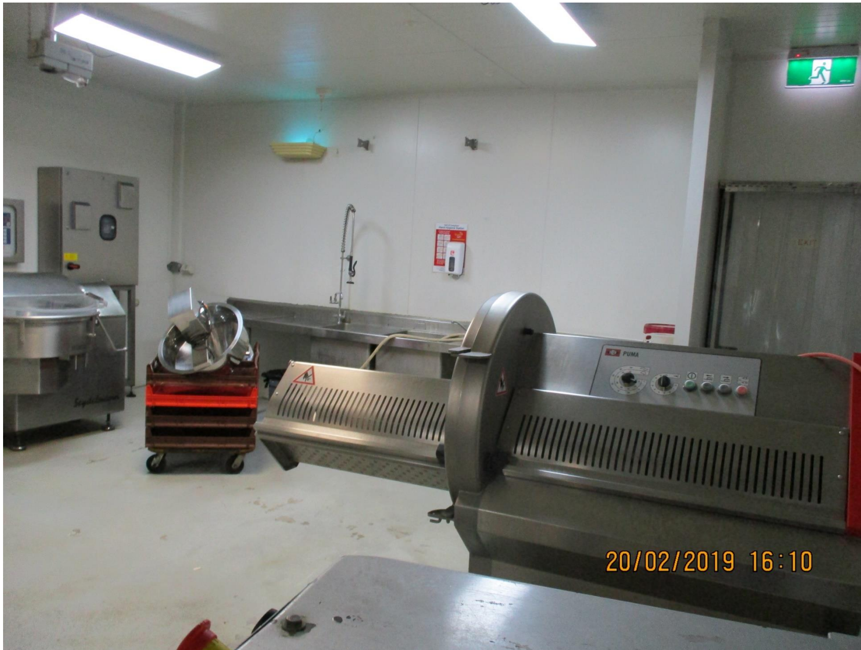
I Cook Foods – Butchery Area photo depicts food processing equipment in close proximity to dishwashing sinks LJ 12
