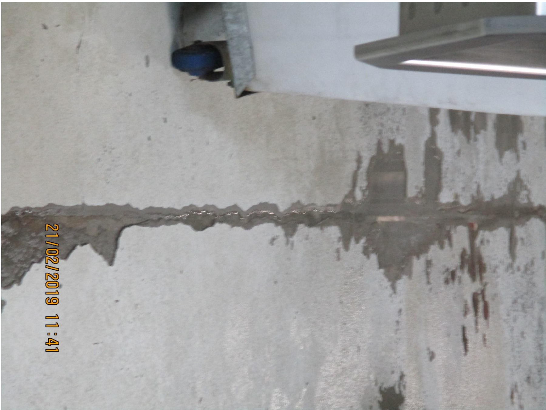
I Cook Foods – Butchery Area photo depicts floor in disrepair pooling water LJ 55
